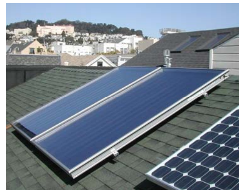
Elizabeth's solar water heating collectors next to her PV panels
